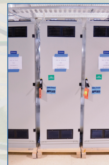
Instrumentation and control (I&C) cabinets for an AP1000 plant
