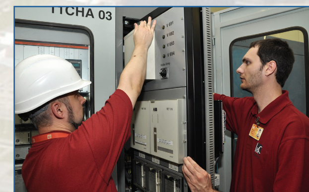
Performing inspection and maintenance on a generator protection system
